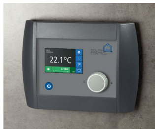
Solar Control Panel
