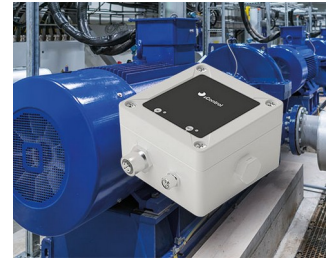
Sensor box for system monitoring
