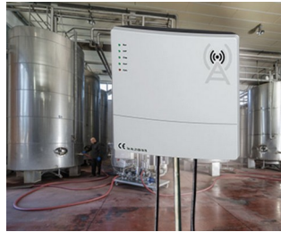
Gateway for the automation of production plants
