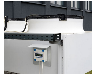
Heating/air conditioning/ventilation control
