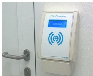
RFID access control readers
