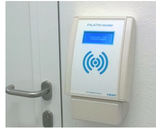
RFID access control readers
