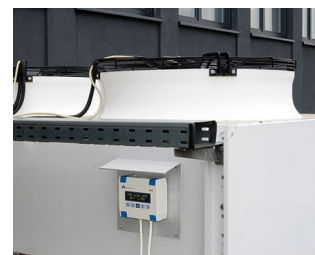
Heating/air conditioning/ventilation control
