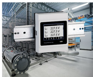
Monitoring of electrical variables
