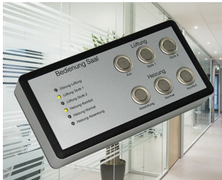
Individual room control panels
