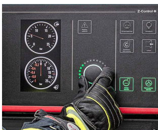
Control element for pump control station
