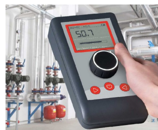
Find compressed air leaks using ultrasound
