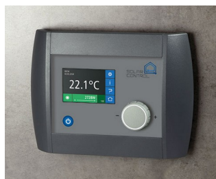
Solar Control Panel
