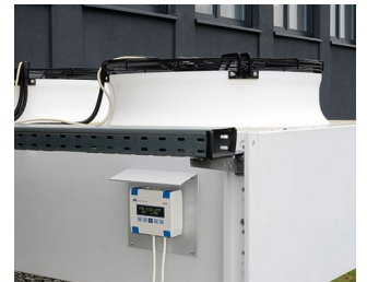
Heating/air conditioning/ventilation control
