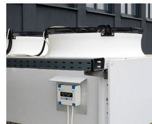
Heating/air conditioning/ventilation control
