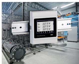
Monitoring of electrical variables
