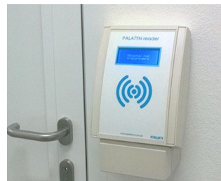
RFID access control readers
